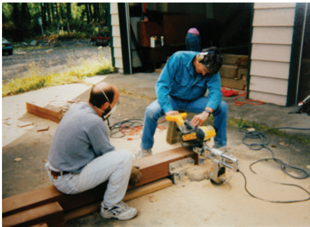
Photo Courtesy of Girdwood Trails Committee Norman Starkey (L) and Tom Yeager (R) work on the timber frame for the hand tram.
